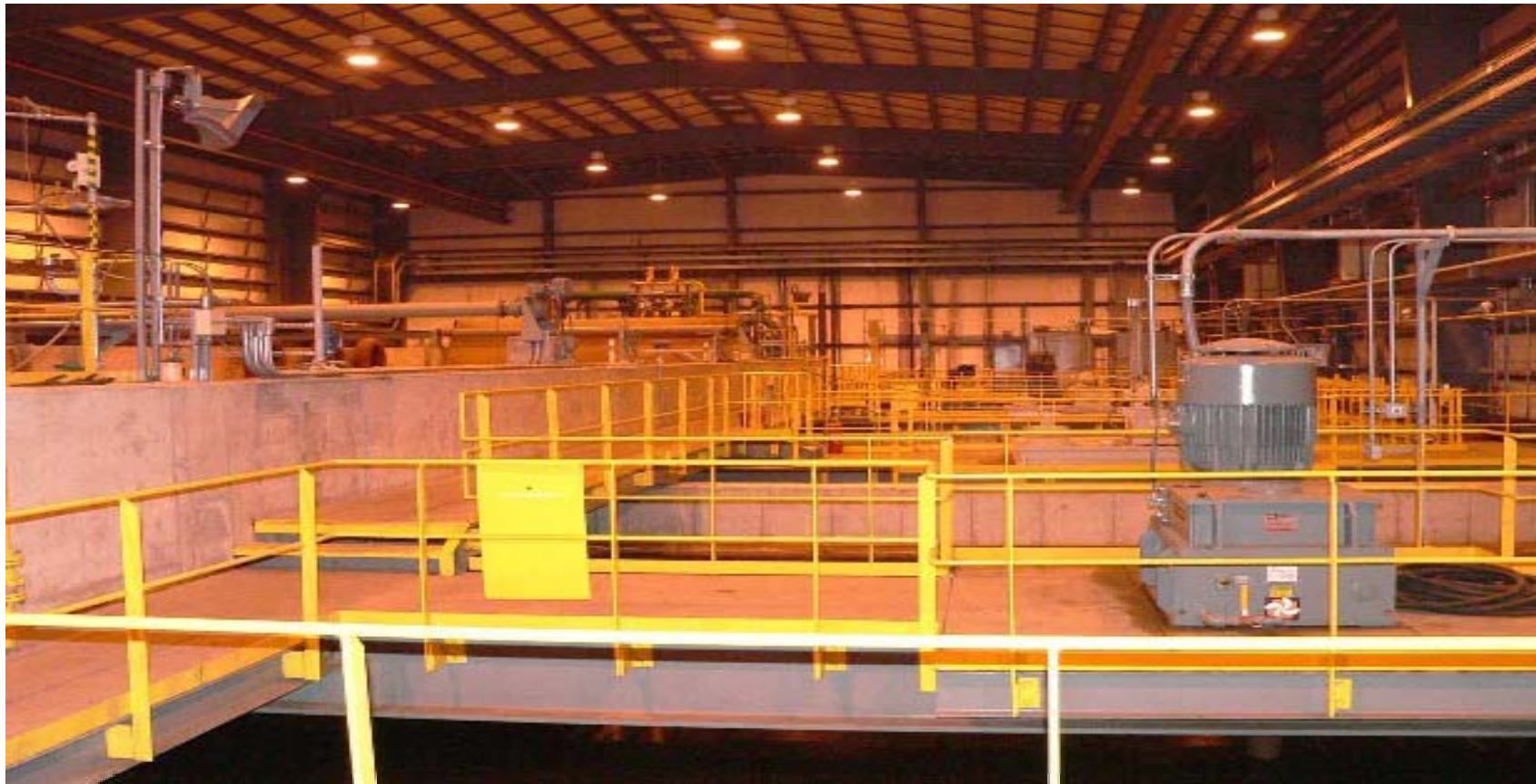
General View of 2 x 17,000 m 3 /h Actiflo Trains
